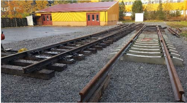
Figure 8 LTU test track
